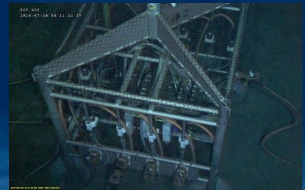
Junction Box (July 2016)
