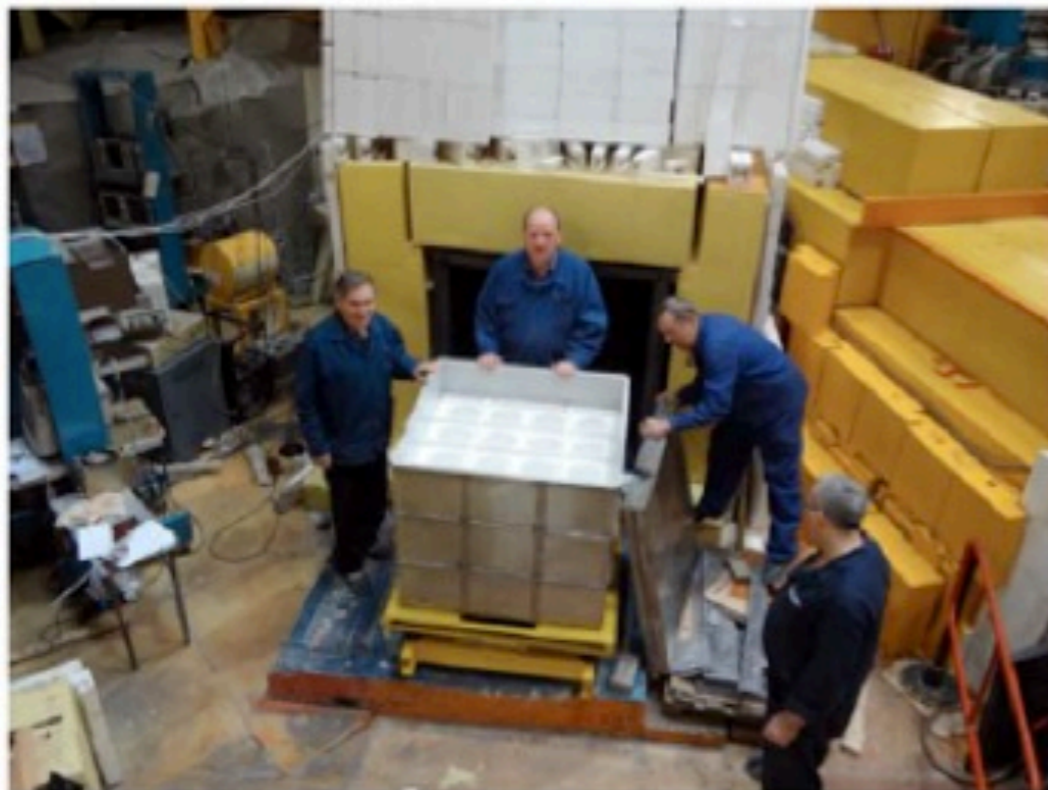
Installation of 2 sections test antineutrino detector with liquid scintillator (total volume 0.4 m 3 )
