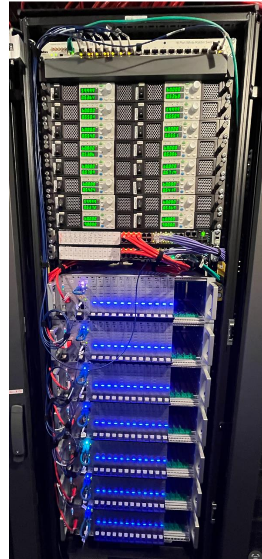
Upgrade rack in ICL
